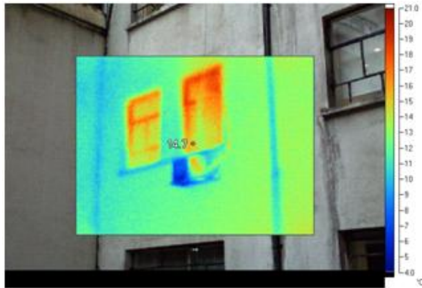
Figure 8: Example of thermal image of uncontrolled heated air leaking through windows.
